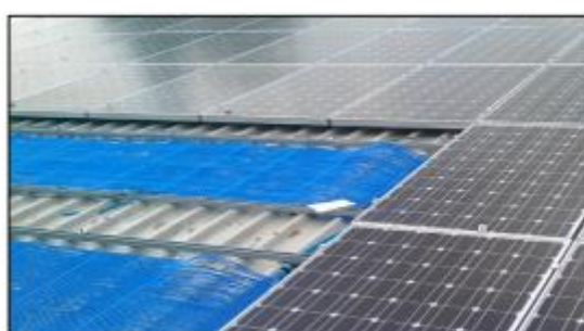
Figure 2 Integration of the poly heat loop underneath PV modules
