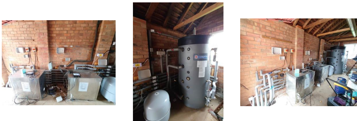
Figure 11 - Installation of the Solar assisted heat pump and the Ground source heat pump at the UK demo building
