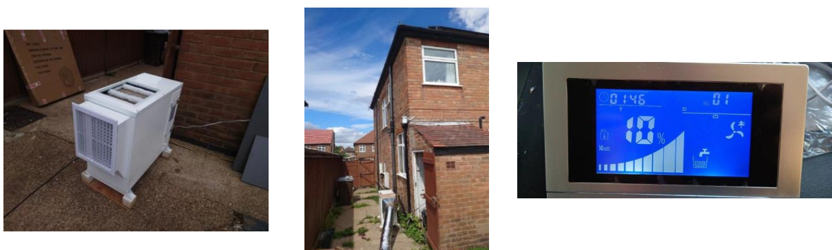
Figure 7 - Evaporative cooler - Installation at the UK demo building
