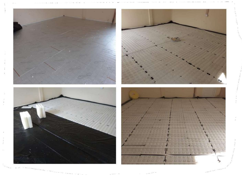
Figure 32 - Underfloor heating installation coupled with PCM
