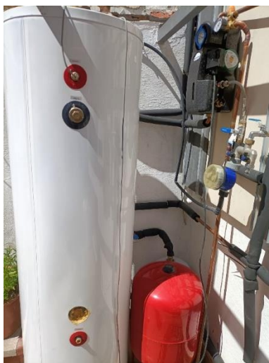
Figure 7 – Spanish building: outdoor installation of the storage tank and auxiliaries
