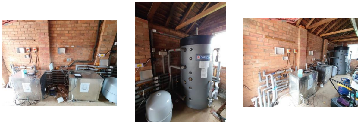
Figure 11 - Installation of the Solar assisted heat pump and the Ground source heat pump at the UK demo building
