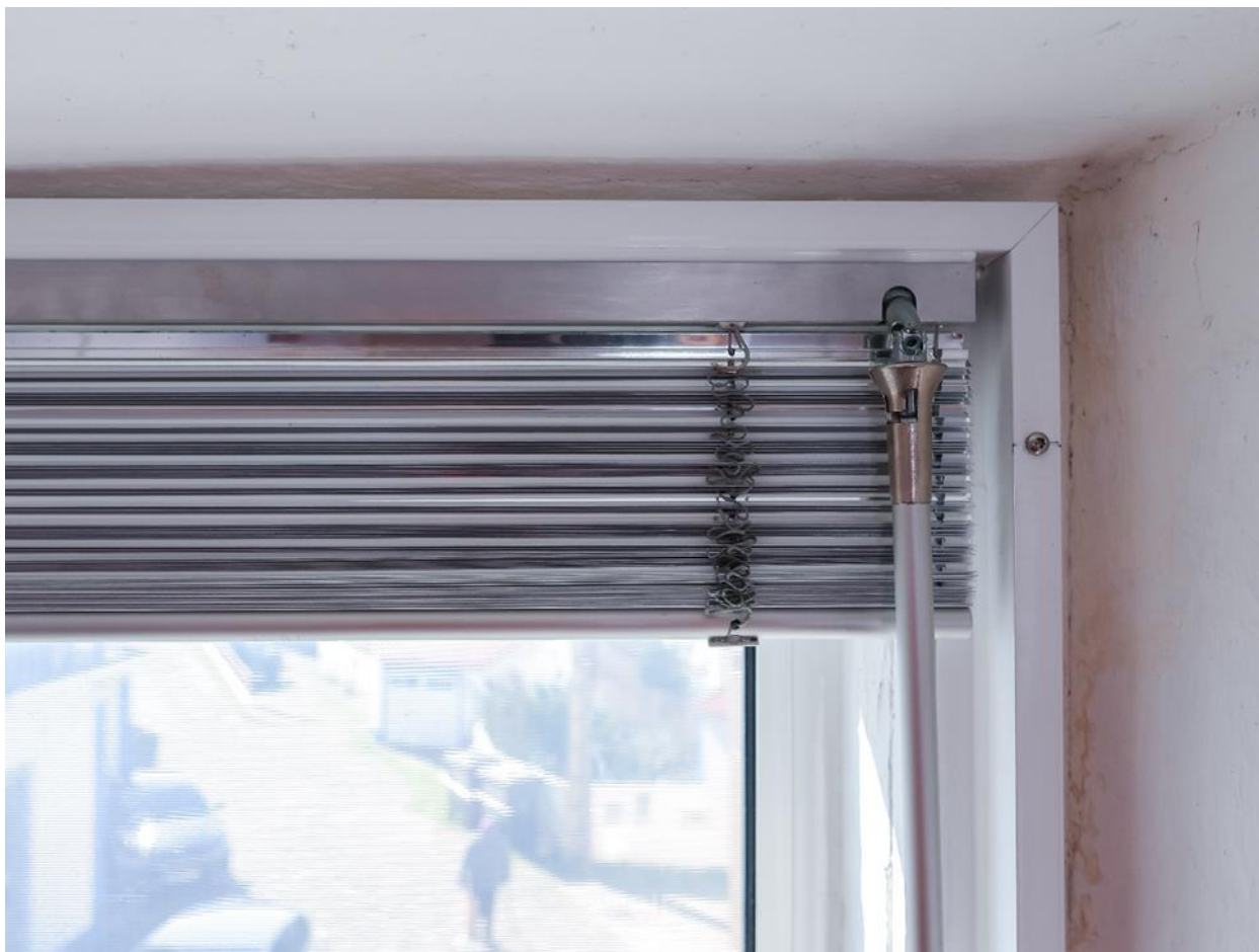
Figure 77 - Daylight Louvers - Portuguese demo case
