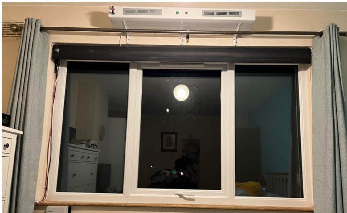
Figure 21 - Integration of Window heat recovery unit with the PV-VG unit inside the bedroom
