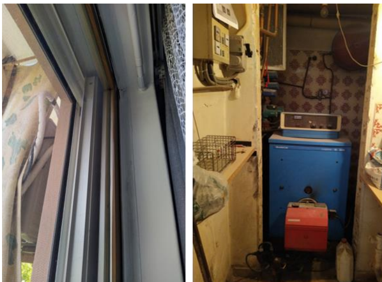
Figure 53 - Old window frame and the old diesel boiler
