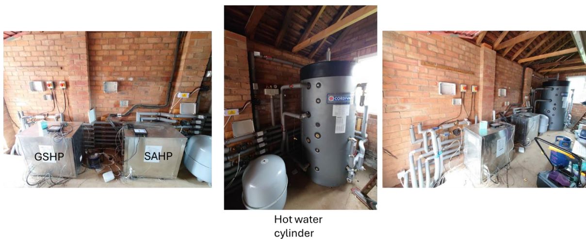
Figure 18 - Installation of both SAHP and GSHP unit and a hot water cylinder inside the garage space
