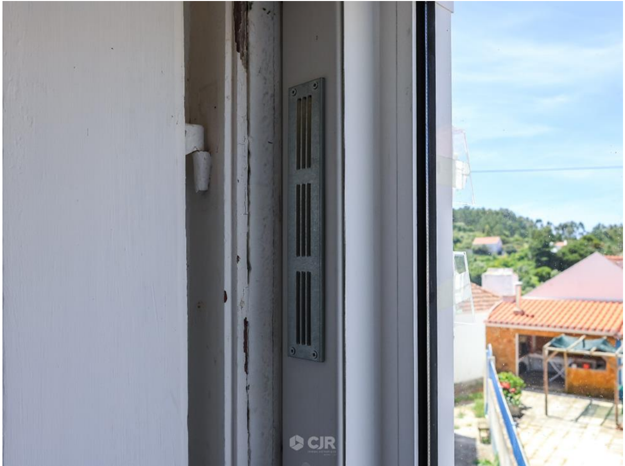
Figure 76 - Window Heat Recovery - Portuguese demo case
