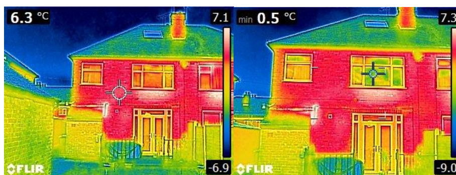
Figure 9 - Thermographic imaging of the back side
