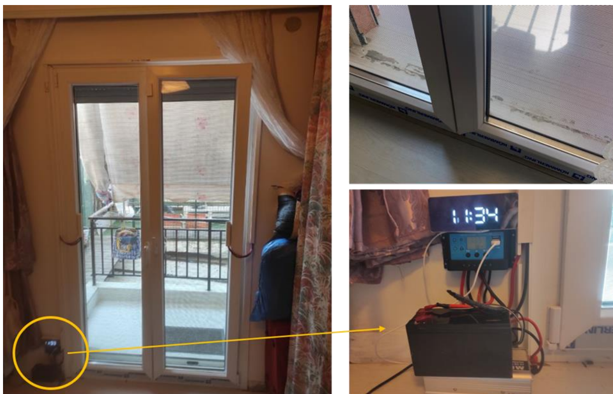
Figure 70 - The PV vacuum glazing installed inside the aforementioned balcony PVC door and the auxiliary devices
